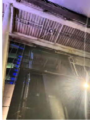
Figure 17 – Non-operational pendant cylinder over elevator
