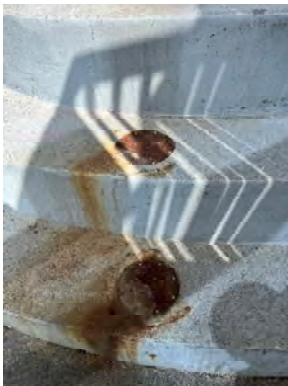
Figure 19 – Rusted in-grade faceplates
