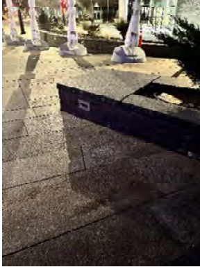
Figure 16 – Non-operational steplights in planter
