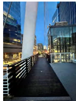
Figure 7 – Non-operational deck lighting
