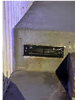
Figure 15 – Non-operational steplight with corrosion
