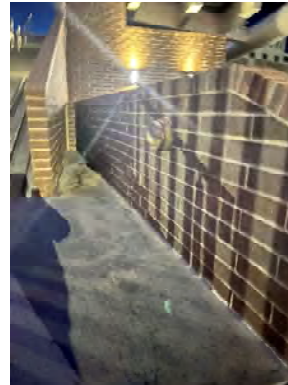
Figure 13 – Non-operational steplight and yellowing lens
