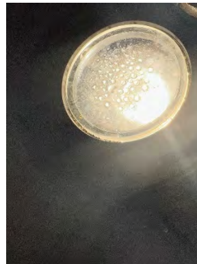
Figure 20 – Flagpole light with condensation inside
