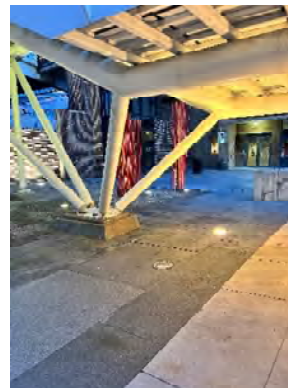
Figure 4 – Stair non-operational in-grade
