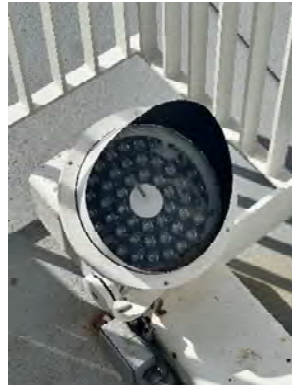
Figure 10 – Mast light with black substance on lens
